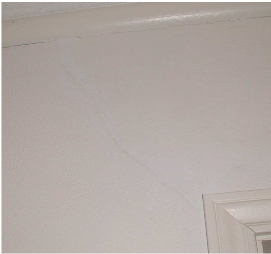
Photo 1: \frac{1}{4} " crack running diagonally from an interior door up to the ceiling.
