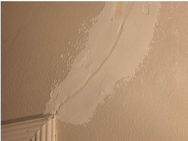
Photos 2 and 3: 1/2" crack that opened and closed. Crack had been filled with compound for over two years and was left unfinished and not smoothed out. Nevertheless, cracks have never appeared within the filled opening.
