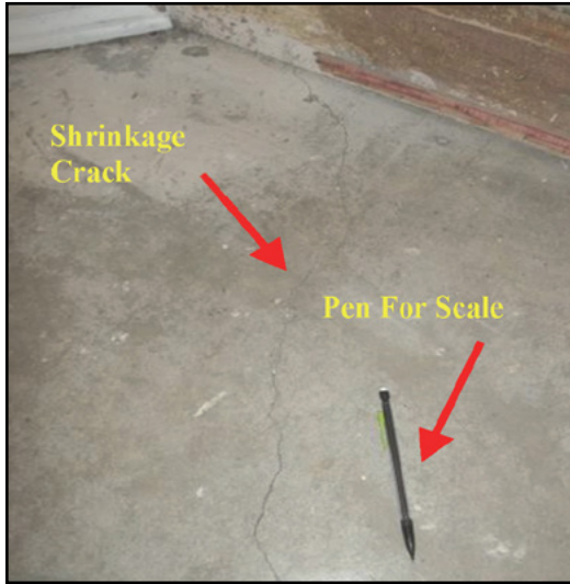
Figure 2-20. Typical concrete crack.
