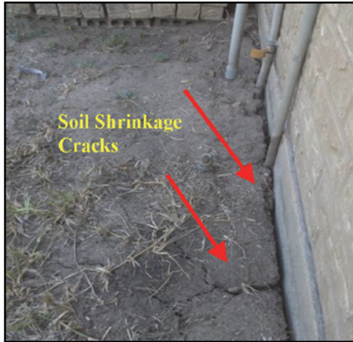
Figure 1-17. Gap caused by soil shrinkage.
