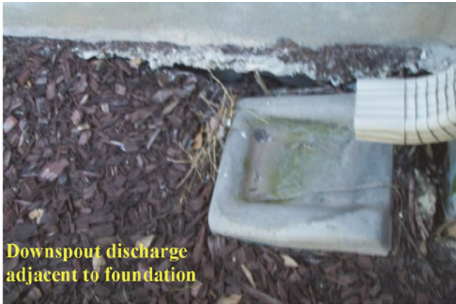
Figure 1-28. Poorly placed downspout.
