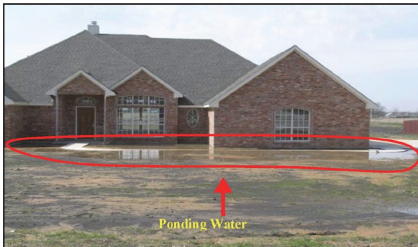
Figure 1-29. Poorly graded site that allows water to pond near the foundation.
