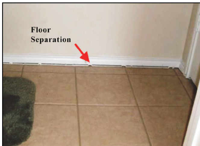
Figure 1-26. Floor/wall separation at perimeter wall owing to center lift.
