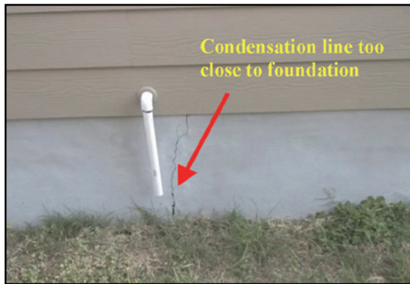
Figure 2-14. Improperly draining air conditioner condensation line.
