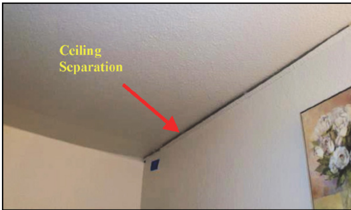
Figure 1-24. Ceiling wall joint separated at the interior partition because of slab edge lift.
